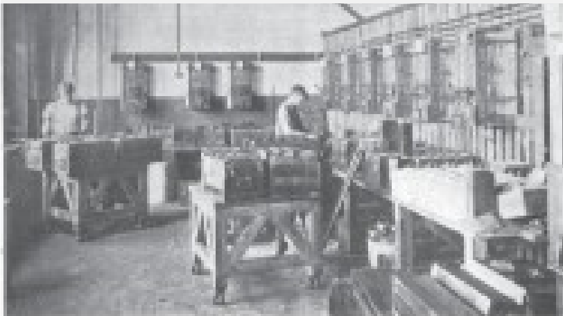
APPROXIMATE BATTERY ROOM
